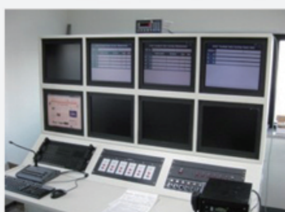
GATE Control Center
