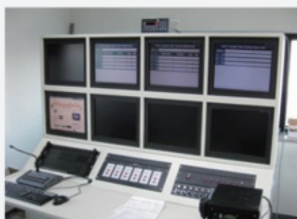
GATE Control Center
